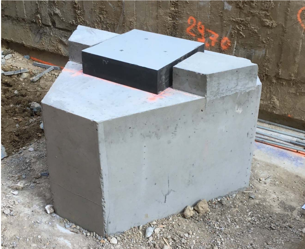
Fig. 8 – Elastomeric bearing pad on top of lower concrete block (Block B)
